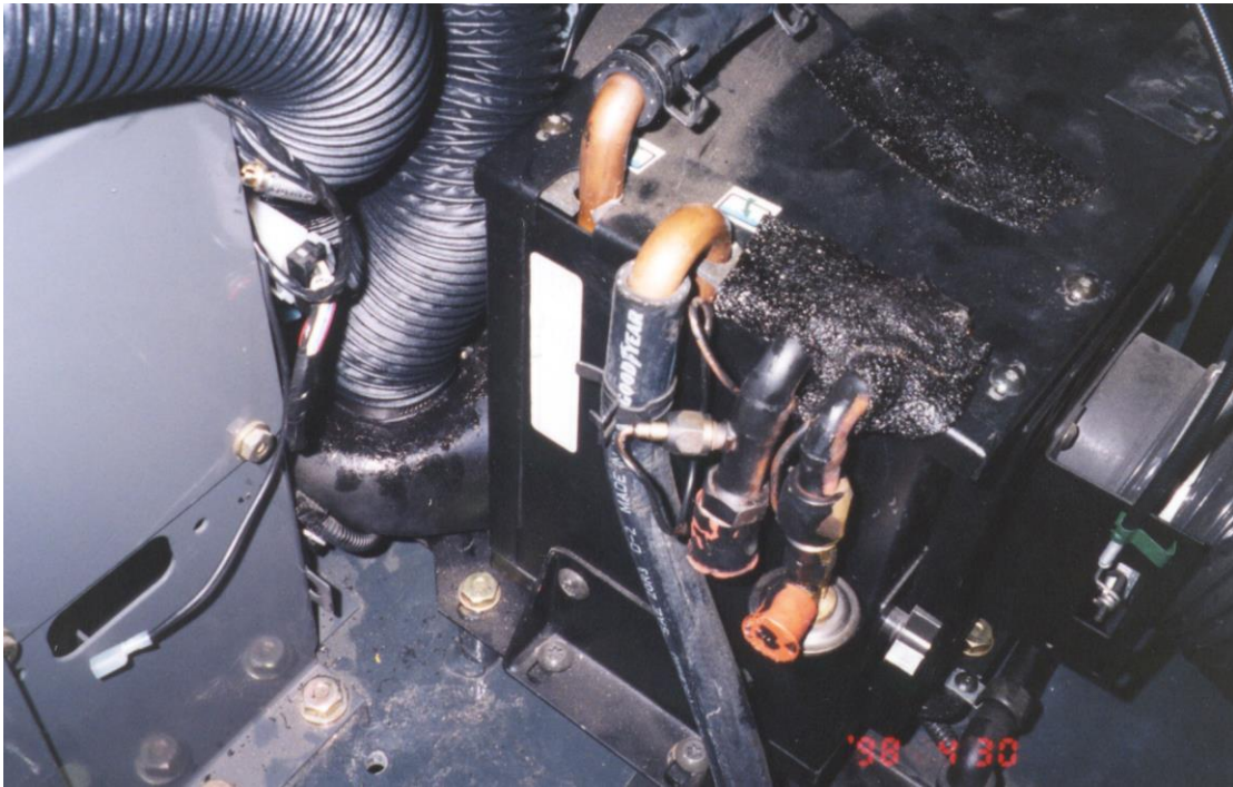
Flex duct connections on outlet air duct.
